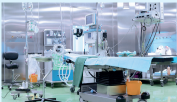
Sealing in operating theatres, medical examination and laboratory rooms
